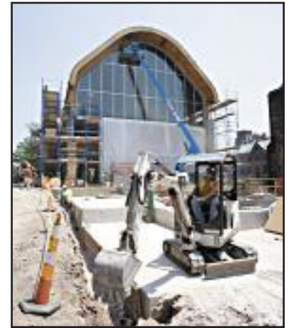
Kroon Hall, a New Haven project for Turner Construction Co., a nationwide contractor with offices in Milford, will showcase the latest developments in green building, combining cutting-edge technology and locally sourced materials.
